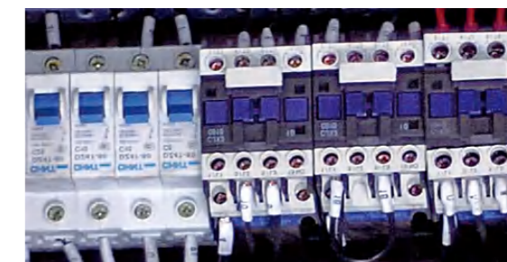
Schneider electric part
